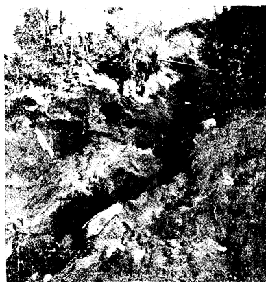
写真 4 岩盤弱線部による崩壊 (北崎村) Phot. 4 Landslide due to discontinuous plane between strong and weak parts in bed rock.
