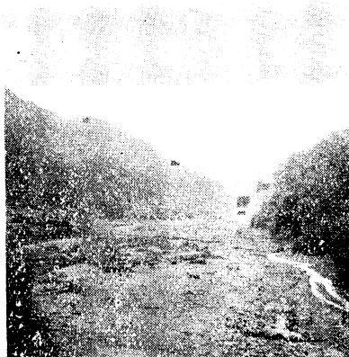
Phot. 62 川床の堆砂 Sedimentat on on river bed
