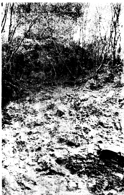
Phot. 7 崩 壊 Landslides.
