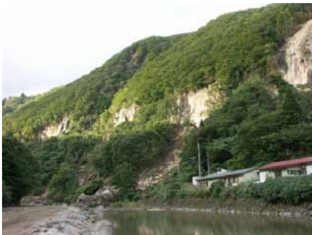
Photo 10. 湯湯付付近に見られるトップリング（北川溶結凝灰岩中の節理の崩落による崩壊）。 Toppling failures occurred along Ichihazama river, because perpendicular joints are well developed in Kitagawa welded tuff. The photo was taken near Nuruyu hot spring.
